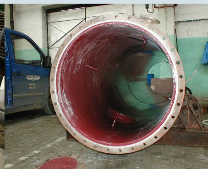
NEUTRALIZATION TOWER LIFE EXTENDED
