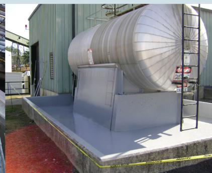
CHEMICAL CONTAINMENT PROTECTED
