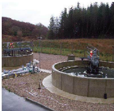
Impact and abrasion damage to concrete clarifiers
