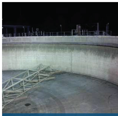
Hard to clean, damaged concrete trough
