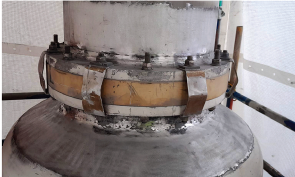
Flange leaking SF 6 gas
