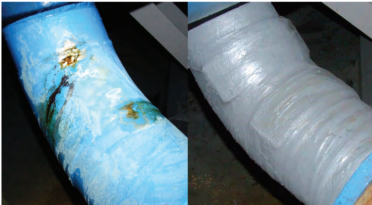
Internal corrosion resulting in pin hole leaks
