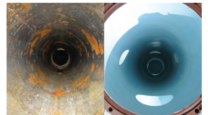
Desulfurization unit protected with coating
