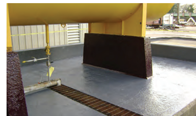
Sulfuric acid containment area coated and protected
