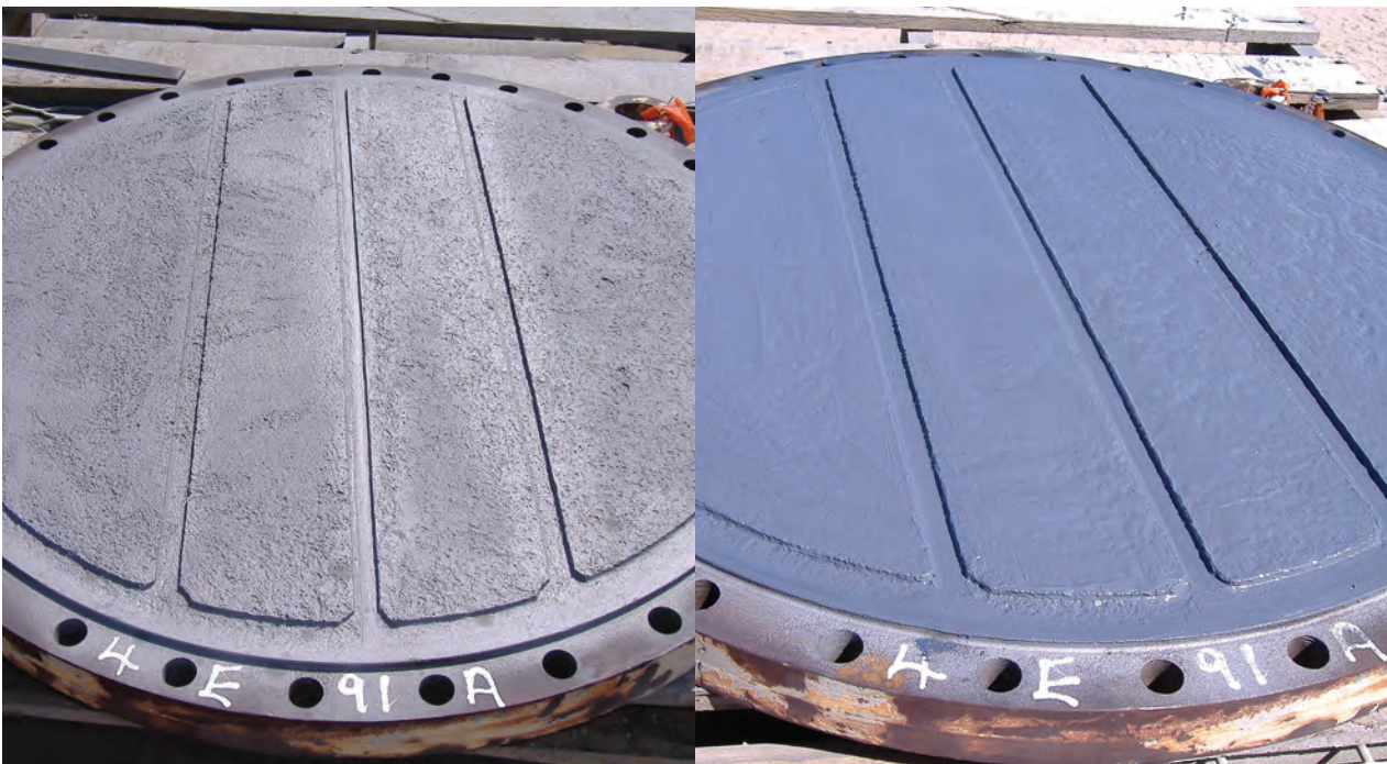
Erosion of thickness and gasket sealing surfaces
