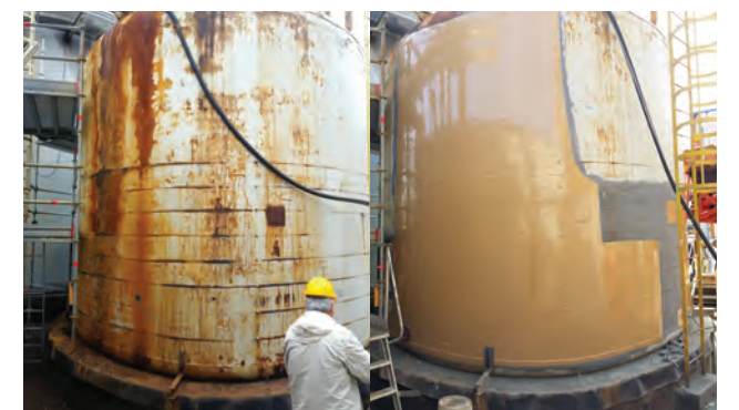
External corrosion protection on tank
