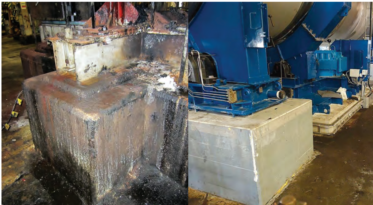
Damaged concrete plinths
