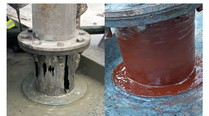
Damaged acid intake nozzle rebuilt
