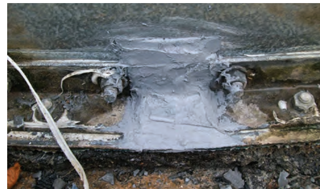
Tank base causing local flooding sealed
