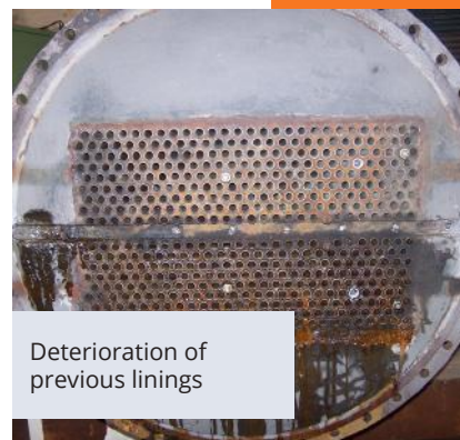
Rapid corrosion to brine heat exchanger
