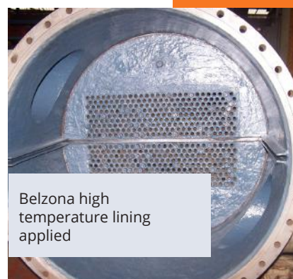
Deterioration of previous linings
